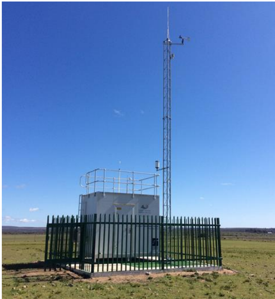
Figure 1.1: Representation of an air quality monitoring station
