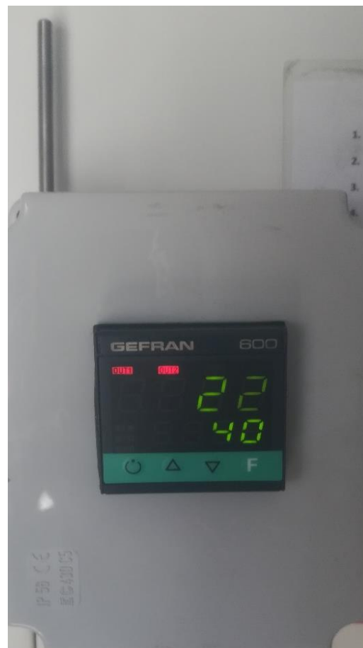
Figure 1.9: Internal temperature sensor is used to monitor the inside temperature of the station.
